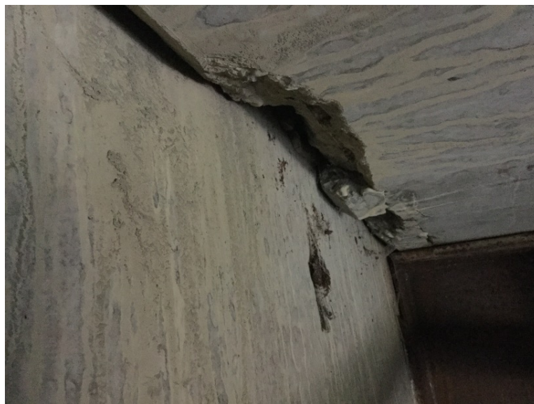
Damage to underside of panel 1 right bank
