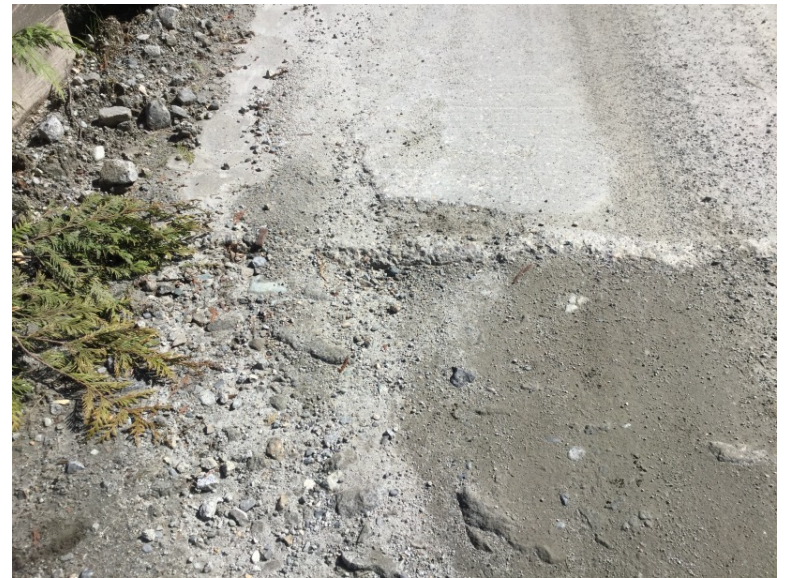
Damage noted to ballast wall and deck panel on wheel path
